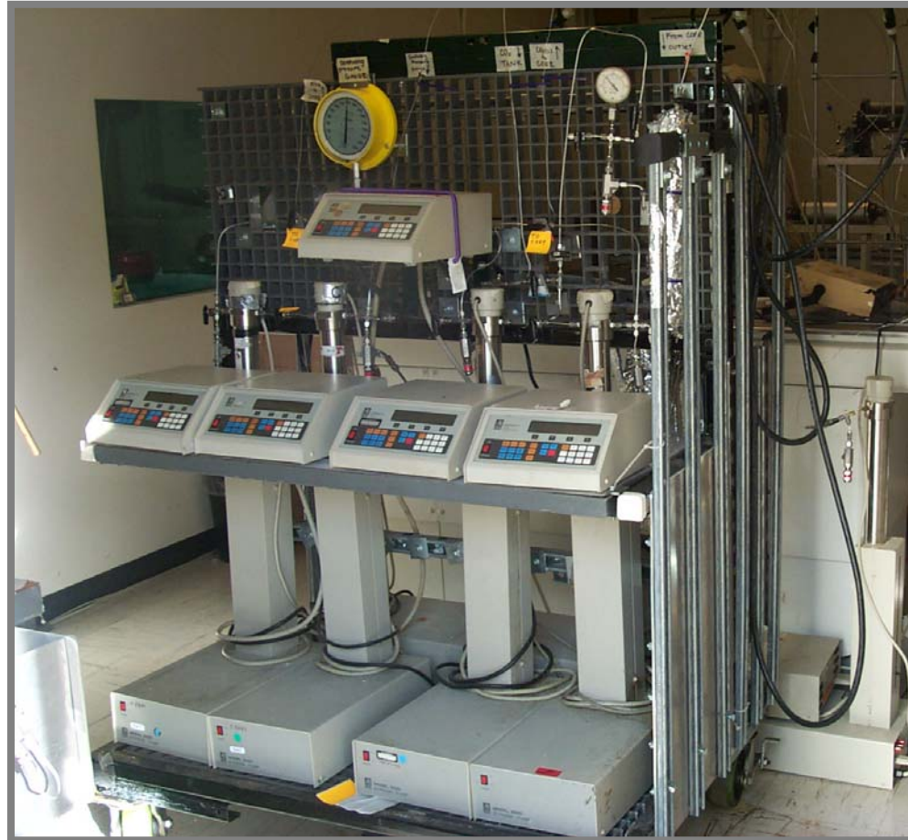
High Pressure Pumps
